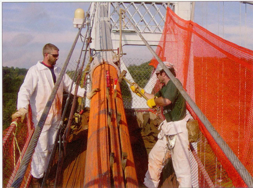
▲ Cable Close-Up. Bridge crews insert wedges to open up a cable in Mid-Hudson River Bridge.
